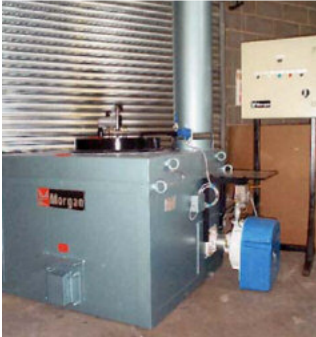
▲ Morgan's Oil Fired Bale Out Furnace.
